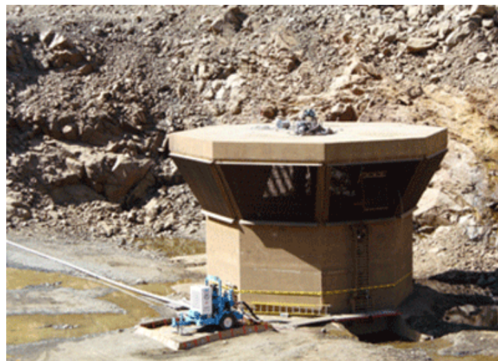
Figure 2. The upper intake, or "mushroom," sits in the upper reservoir of the Cabin Creek facility. Source: CSB
