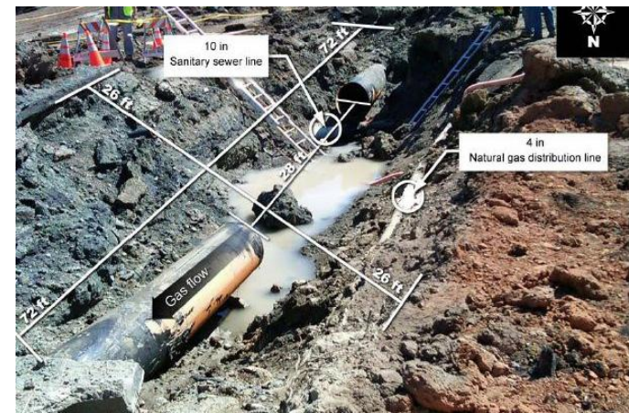
Figure 1: The ruptured segment of pipe, discovered 100 feet away from the crater, was 28 feet long and weighed approximately 3,000 pounds.
