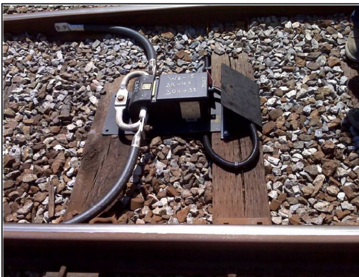
Figure 2: Each impedance bond acts as a transmitter for one track circuit and a receiver for the adjacent track circuit.
