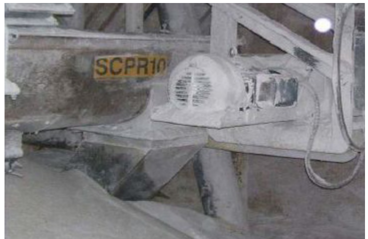
Figure 3: Imperial Sugar photo taken in the Fall of 2006 showing machinery, floor, and architecture covered with sugar. The coated machinery would sometimes overheat and ignite the surrounding sugar.
