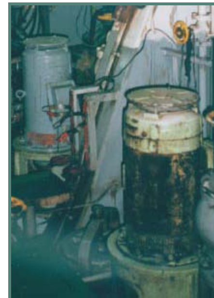
The Bright Field's #1 and #2 engine oil pumps
