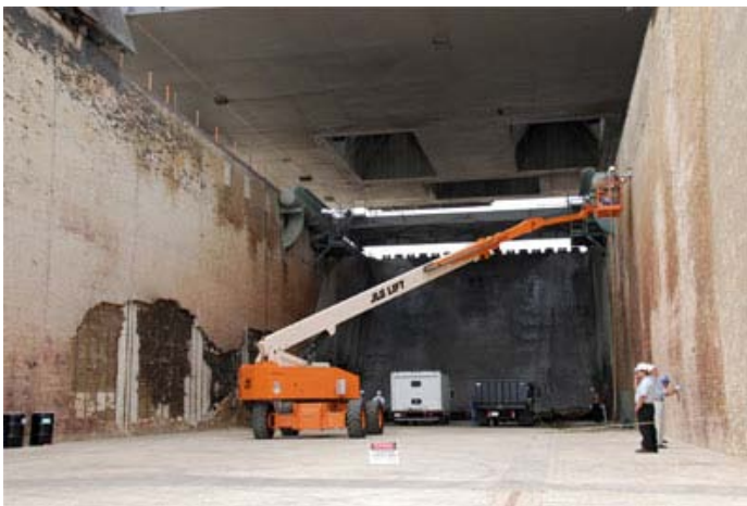
Figure 4: Workers strip loose bricks from the flame trench wall for the Fondu Fyre application.
