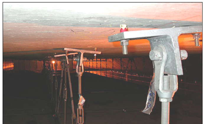
Figure 4: Numerous anchor bolts were found to have been affected by creep.
