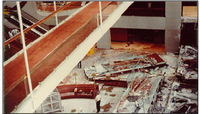
Figure 1: Pieces of the collapsed walkways in the atrium.
