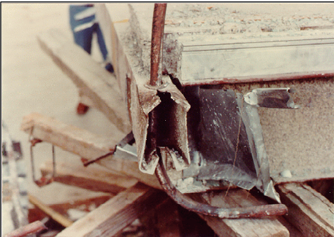
Figure 4: Ruptured box beam on the collapsed walkway.
