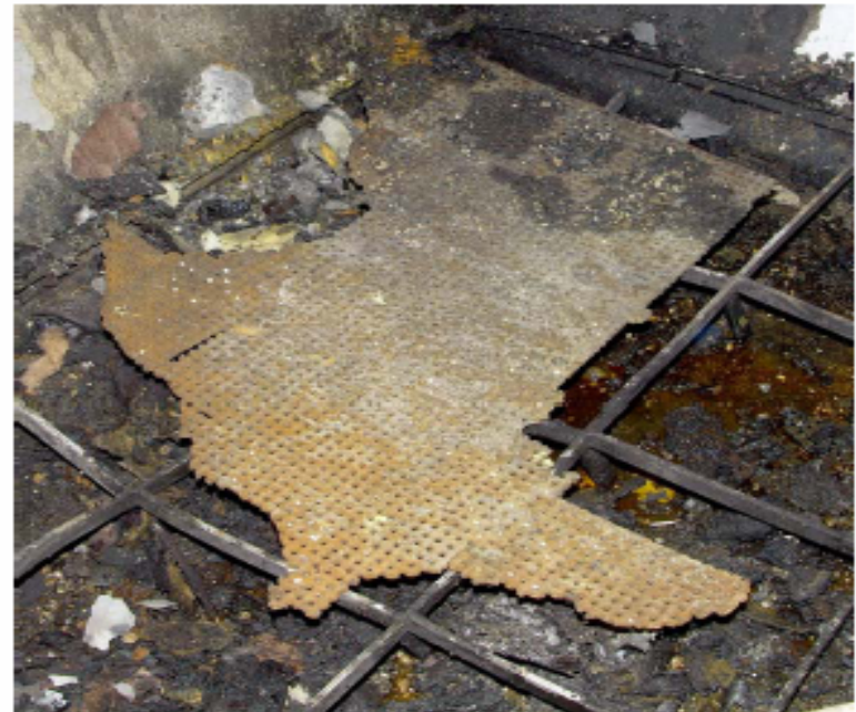
Perforated Filter Bed
