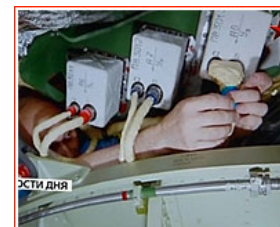
A trio of angular velocity sensors, DUS on their mounting platform (top) and their installation on the rocket. Credit: Zvezda TV channel
