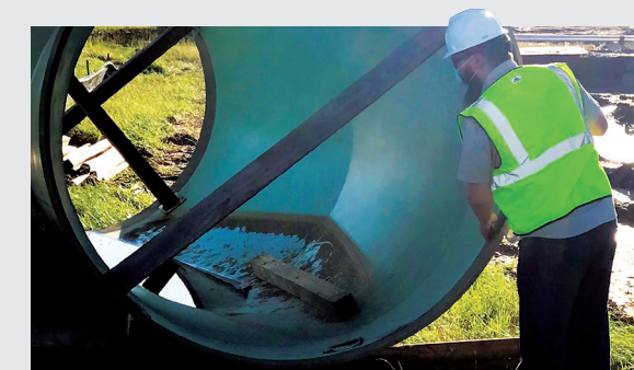
Stennis Space Center: An S3 contract engineer performed an inspection of a 75-inch mitered pipe elbow, which will be installed on the High-Pressure Industrial Water A-Complex pipe.
