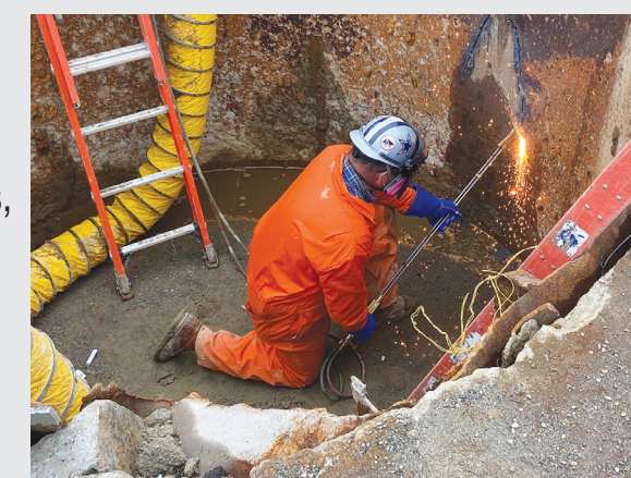
Glenn Research Center: Larry Idler performed torch cutting work in a confined space with safe work practices, including ventilation, a respirator, proper egress, flame resistant clothing, air monitoring and other Personal Protective Equipment.
