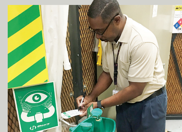
Johnson Space Center: Darvon Collins performed the weekly inspection and activation on a laboratory's plumbed eyewash and shower unit.
