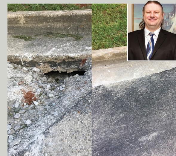
Marshall Space Flight Center: Christopher Tyler initiated the repavement of a parking lot after he identified a section where the earth had been washed out under the pavement and curb at a gas line.
